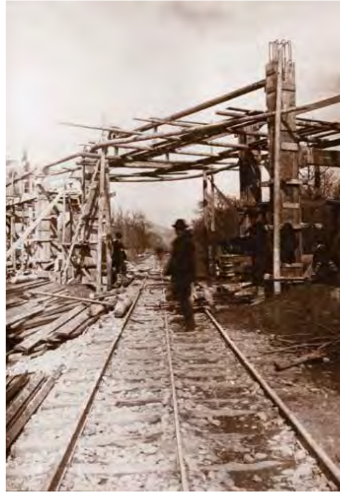
Conduit of the water channel constructed up until 1920, through which the waters of the lalomița River were conveyed to the I. M. Voith turbines
